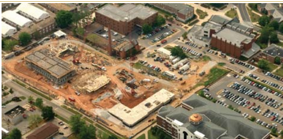
This aerial view shows the large scale of Auburn’s new Transportation Technology Center, which is rising along Magnolia Avenue between other buildings of the Samuel Ginn College of Engineering at the top left of the photo and the College of Business, which is housed in the Lowder Building, one of the larger academic facilities on campus, at lower right. The first phase of the project, budgeted for $54 million, will provide a home for work in several departments in connection with the development and study of advanced technologies in transportation.
