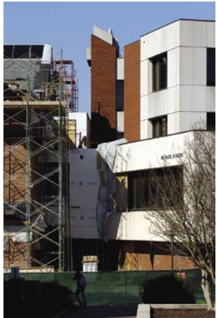
As the new south wing of the W.W. Walker Building takes shape, construction crews work on the connection between the pharmacy building and the 44,000-square-foot wing. A wing on the north side of the building will add another 9,900 square feet.
