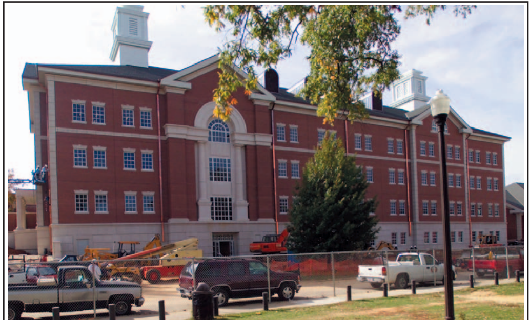
The main building of the Sciences Laboratory Center is in the final stage of construction and is scheduled for completion early next year. The $39 million complex will be the site of most lab courses in AU's core curriculum and will provide modern facilities for advanced research in the College of Sciences and Mathematics and related fields in other colleges at Auburn.
