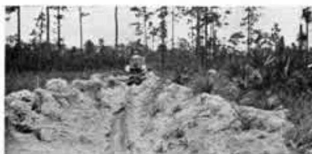
FIG. 12. THE FLORIDA FOREST SERVICE PLOW CONSTRUCTING AN EIGHT-FOOT FIRE LINE IN ONE TRIP. During the years 1933 and 1934, the Forest Service, CCC camps, and landowners plowed or reworked a grand total of 13,465 miles of fire lines or an average of 7.1 miles per section of land.
